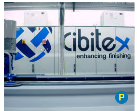
P. Main switch cabinet
