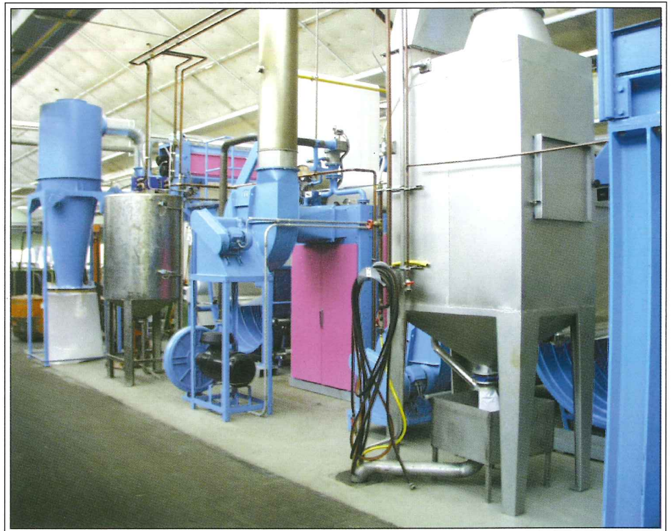
气旋式过滤器、化学液准备槽、水洗过滤单元、鼓风机和吸烟电机 Cyclone filter, chemical tank, air blower, exhaust fan and air washer.
